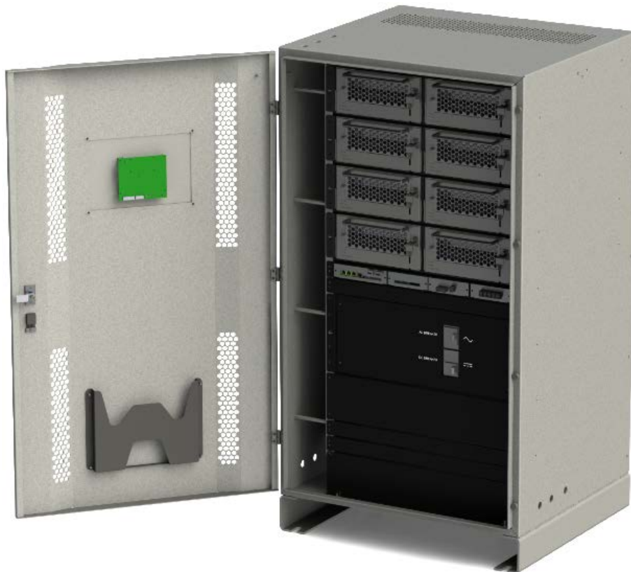
Figure 8. 56 kW battery charger with multiple rectifier modules
