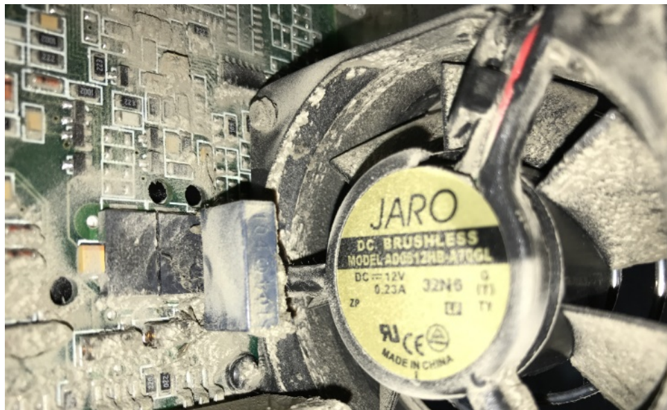
Figure 7. Significant dirt accumulation inside fan cooled inverter after 5 years
